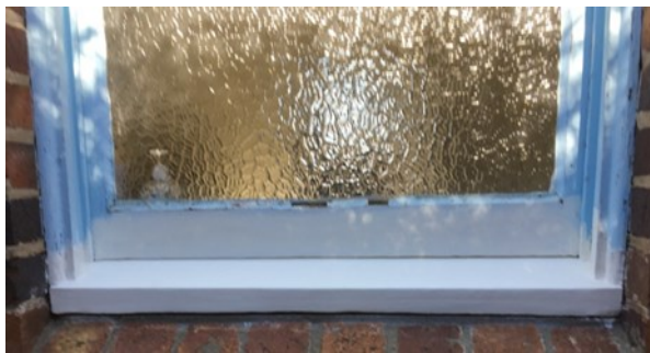
The window sill before and after
