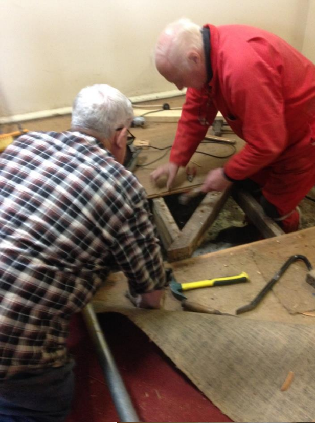
Peter Gitsham and Bruce McMaster removing the floorboards to lower the floor.
